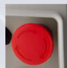
Emergency stop Interruptor emergencia
